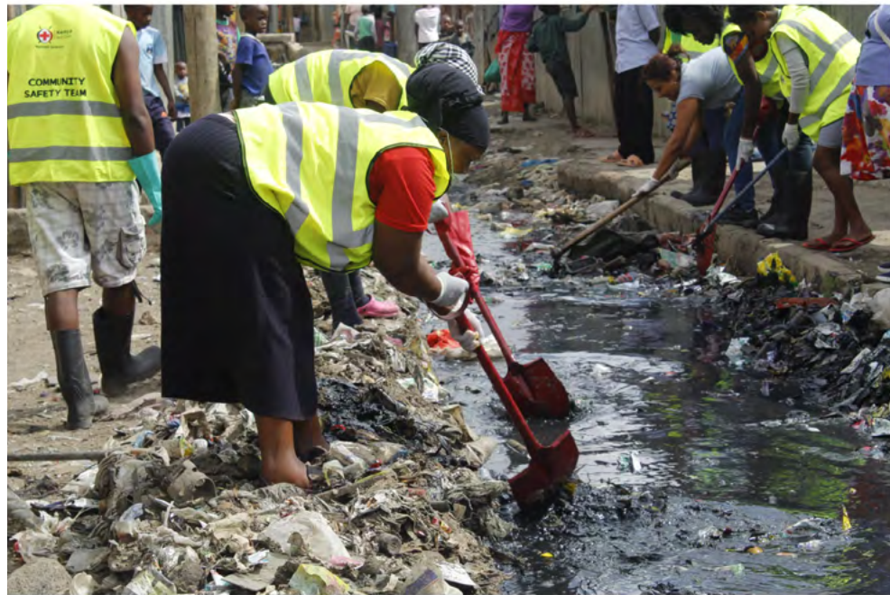
Mukuru Kwa Reuben residents and Muungano federation members from across Nairobi unblocking one of the neighbourhood's drains. Source: Muungano Know Your City TV
