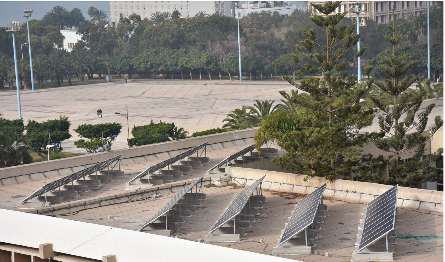
Figure 19. PV Hotel de ville. Source: Municipality of Agadir (2023)
