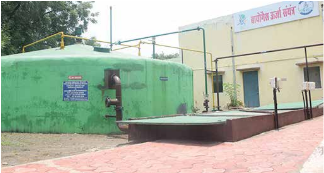
Image 3: A waste-to-energy bio gas plant established by the city.
