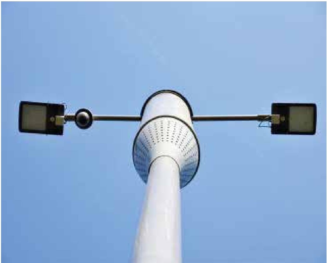
Image 14: A 'Smart Pole' installed in Bhopal that facilitates several utility and connectivity services.
