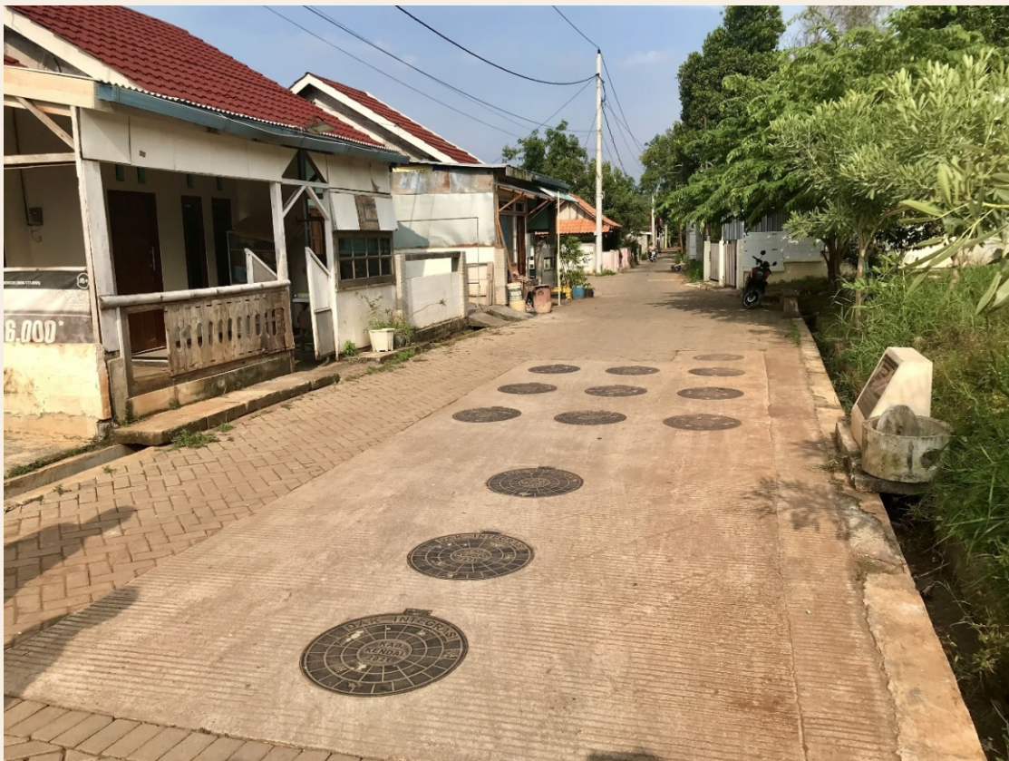
Figure 95. IPAL of the Communal Community Housing of Penyangkringan Village (Source: author documentation)
